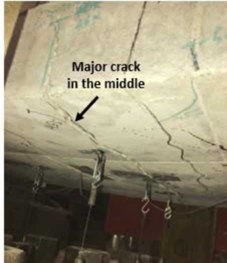
Figure 3-20. Major crack in mid-span of the wall
